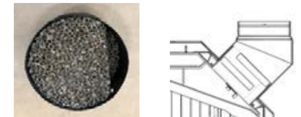
Catalyst installation seen from the flue outlet above the vermiculite smoke baffle plate.
